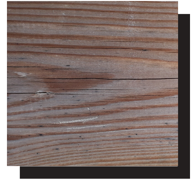
Old wood: after more than 1 year
