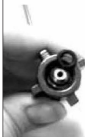
CO2 line to regulator
